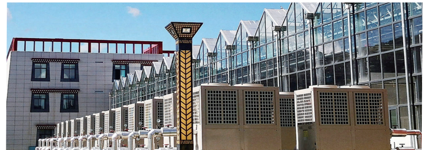
Heat Pump Project, Jingtu Industrial Park in Caina Town, Tibet
