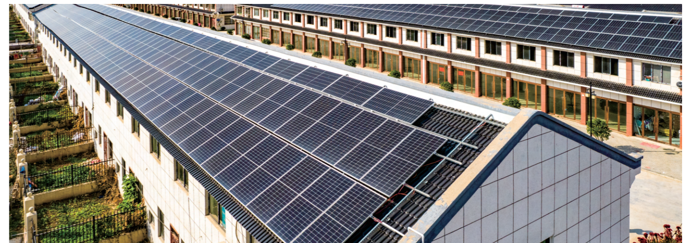
202MW Distributed PV Project (Phase I) of Guannan County, Jiangsu
