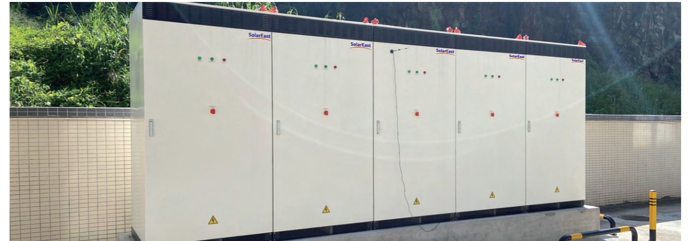
Industrial & Commercial Energy Storage Project, Guangdong
