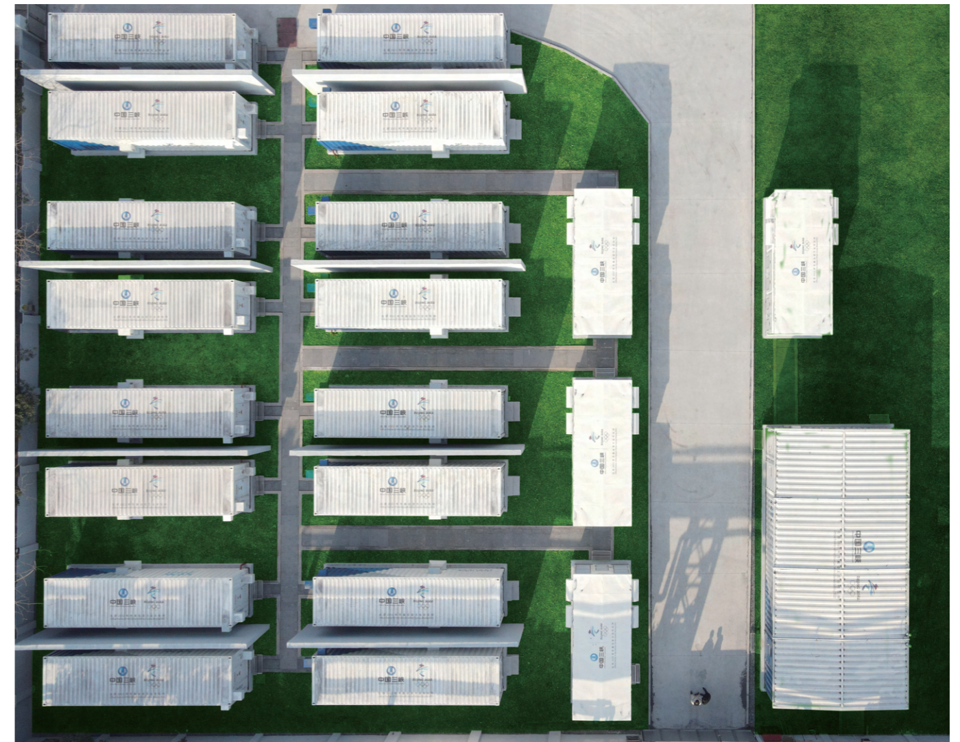
10MW/39MWh Energy Storage Station
